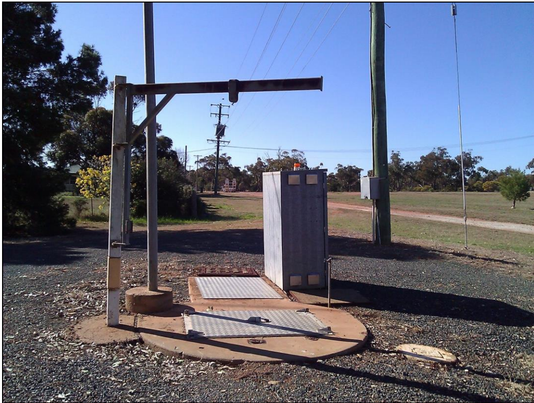
Figure 4.3 - Photo Moulder Street SPS
