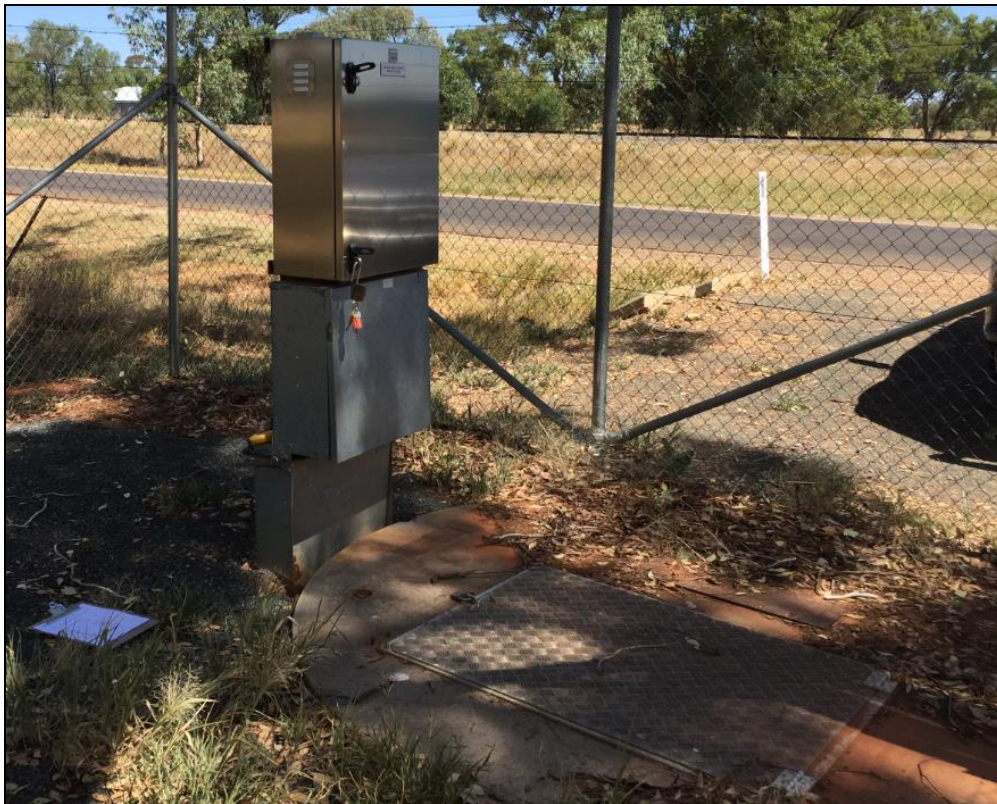
Figure 4.8 - Photo Boona Road SPS
