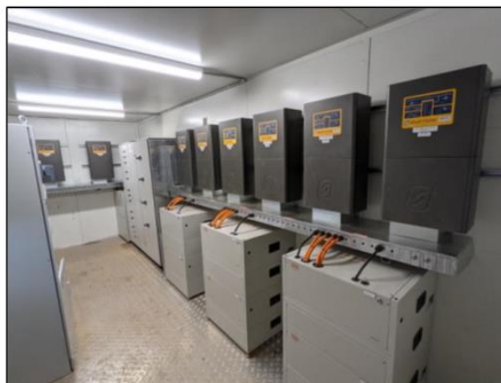
Figure 4: Lake Cargelligo WTP Battery
