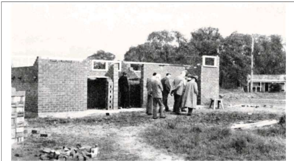
Figure 9: Members of the AWB inspect a new ablutions block being built on the Condobolin Reserve in 1963 (Source: Dawn Magazine September 1963).
