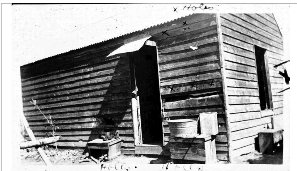
Figure 5: A weatherboard hut at Condobolin Reserve c1940. The photograph was taken by the AWB as part of the inspection of houses and amenities at the reserve site (Source: AWB Collection State Archives and Records Authority [SARA]).
